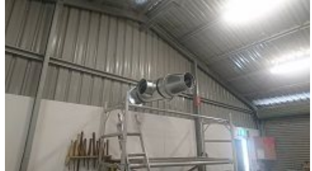
The beginning of the extraction system..
